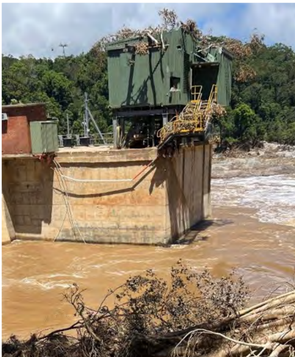
DAMAGE TO KURANDA WEIR. P. Credit CLEAN Co
